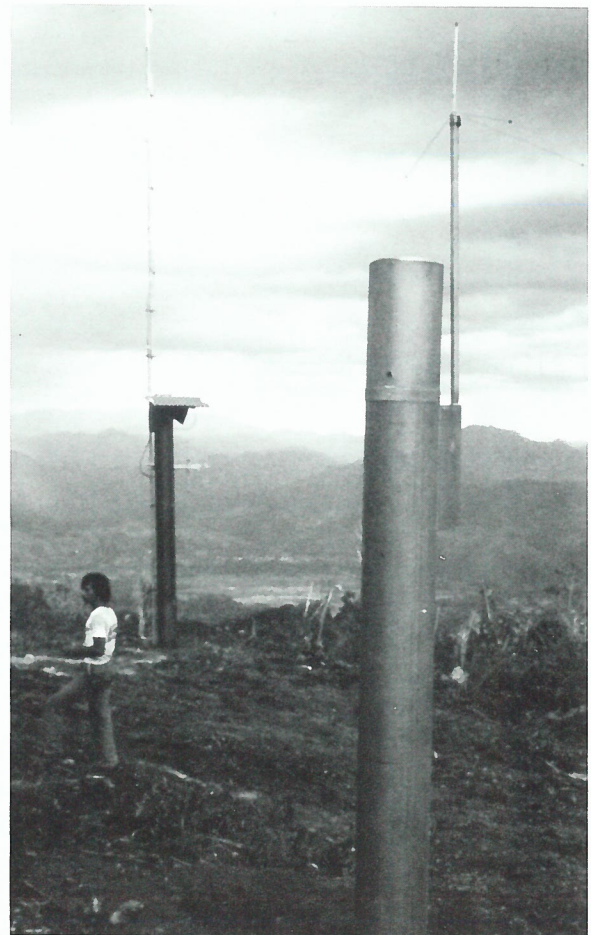
Packaged Repeater Station with Rain Gage in the background, Philippines
